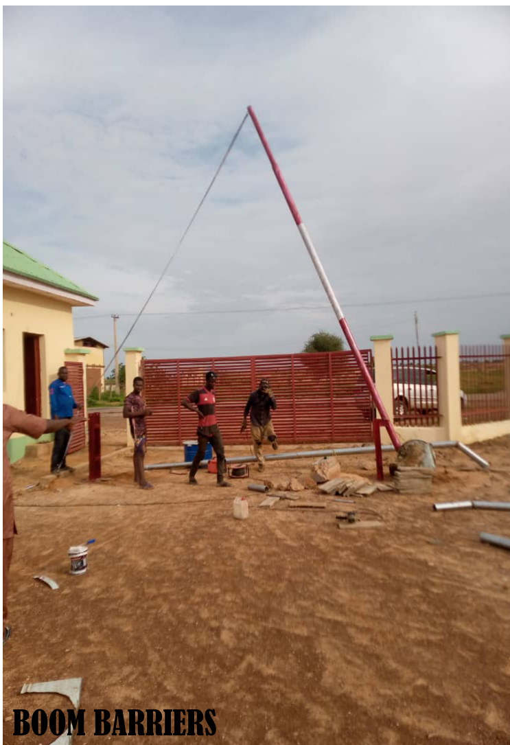
BOOM BARRIERS AT GORONYO
